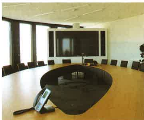
[Top to bottom] Executive meeting room; Presentation tools include Wolfvision visualisers; Videoconferencing is handled by a Cisco codec; and a number of Panasonic 103" displays were installed.
